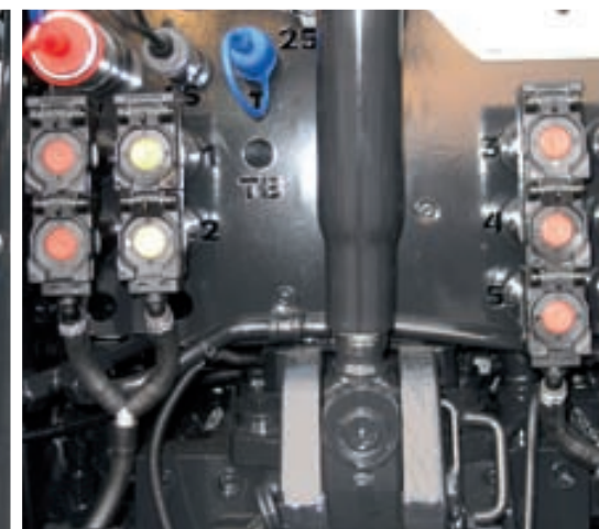
Logically numbered: The hydraulic connections at the rear.
