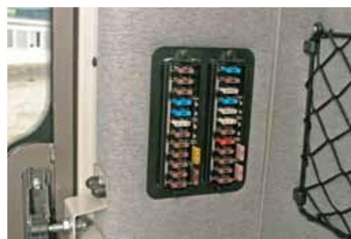
The electrical fuses are in the cab and are easily accessible without physical contortion.
